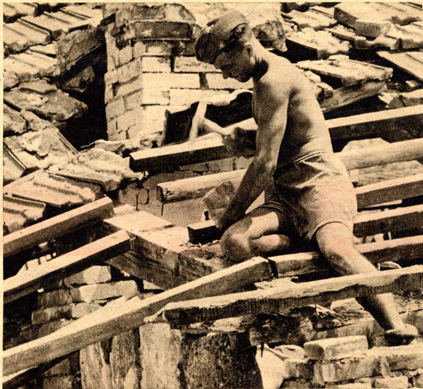
Not a drop of rain falls during the hot season, but that is just the best time to repair a roof, so as to be dry when the fall rains set in
