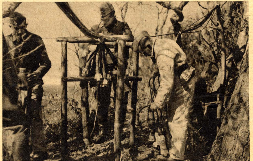
Here can be plainly seen the connections of the numerous cables that converge here in a distributing station. The least slip might spoil the connections, so that the utmost care must be taken
