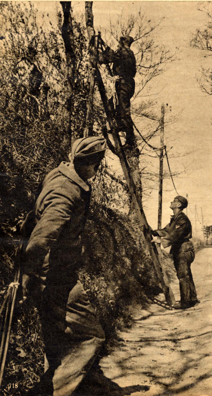
Left: Laying the cables between masts is always a ticklish job, but must be carried out smartly, in spite of that, because the laying of field telephone cables is always done in a hurry
